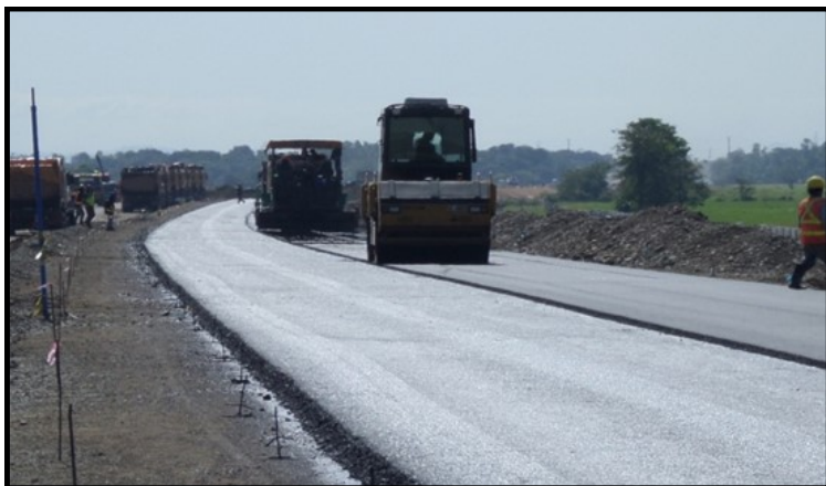
Laying of Binder Course at Sta. 72+400 to Sta. 72+880, SB, CMPCI Photo Source: DPWH Region 1
